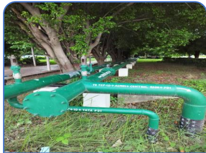
Shifting to over-the ground pipe line from existing under ground pipe lines
